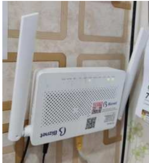
Gambar 34. Access point (Sumber: CV. Hamim Group, 2024).
